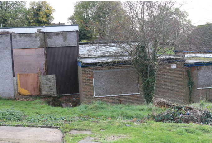
Rear of building – boarding is regularly pulled down
