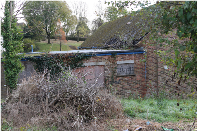
Rear of building with debris that has been there for months
